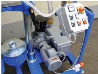
DETAIL OF ELECTRIC PANEL AND VACUUM PUMP
